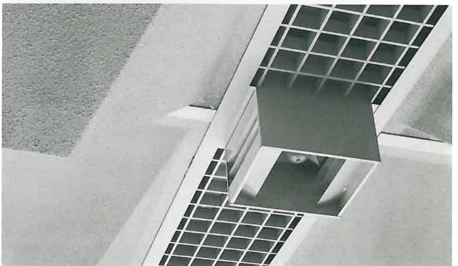
The ceiling of the entrance-hall is made up of fibre-glass coffers mounted on a heavy aluminium framework which also supports the lighting fittings, a detail of which is shown below.
